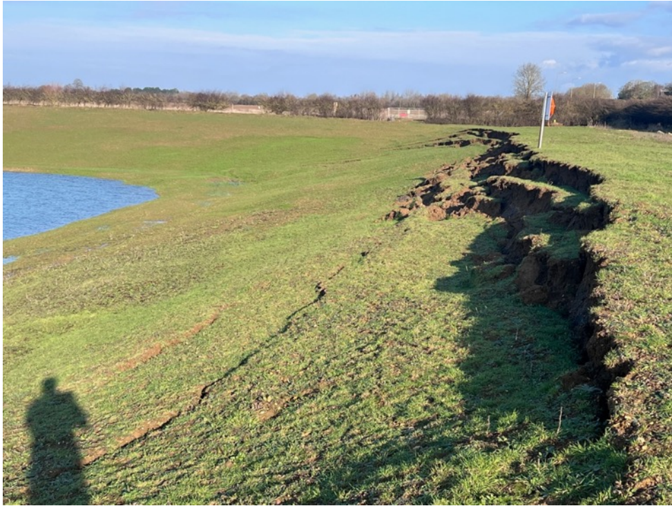
Fig 1: Restoration subsidence in the fields immediately north of the A1175
